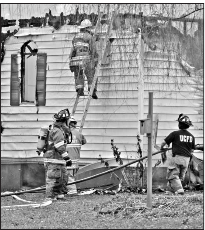
Union County firefighters seek to control hot spots at last week's fire on Ivy Log Creek Lane. Photo/Charles Duncan
