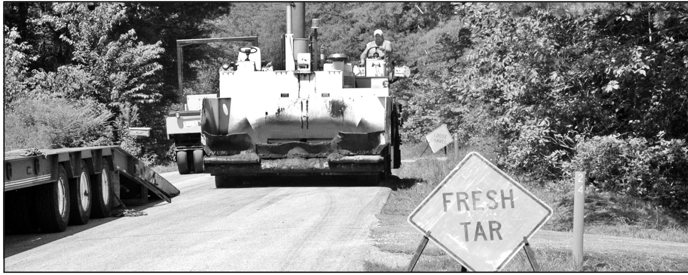
Colditz Trucking has been busy the past few weeks as they work to complete the four miles of paving that they received the low bid on. The money to pave several roadways including Mulkey Gap and Loving Road came via grant dollars to the county. Photo/Todd Forrester
