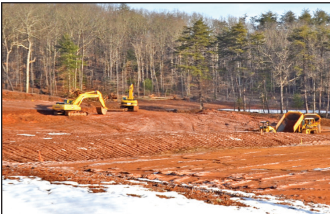
Construction on the new Union County Schools Ag Center began in November, and should be done by the end of the school year
